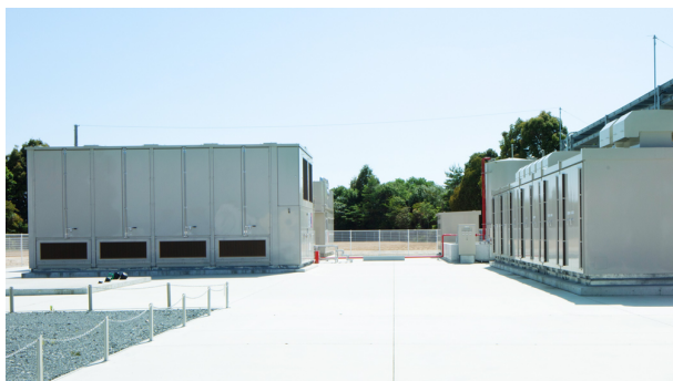
Large-capacity power storage system (Yamaguchi Plant)
