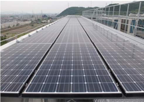
Solar panels (Minase Research Institute)
