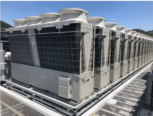
Module-type heat pump chiller (Minase Research Institute)
